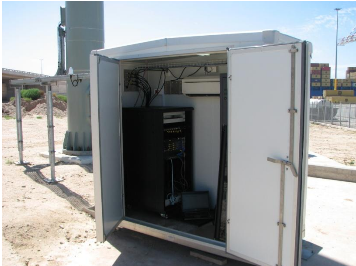
Base Station Container
