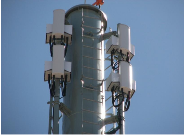
30m Mast with ODU & Antenna
